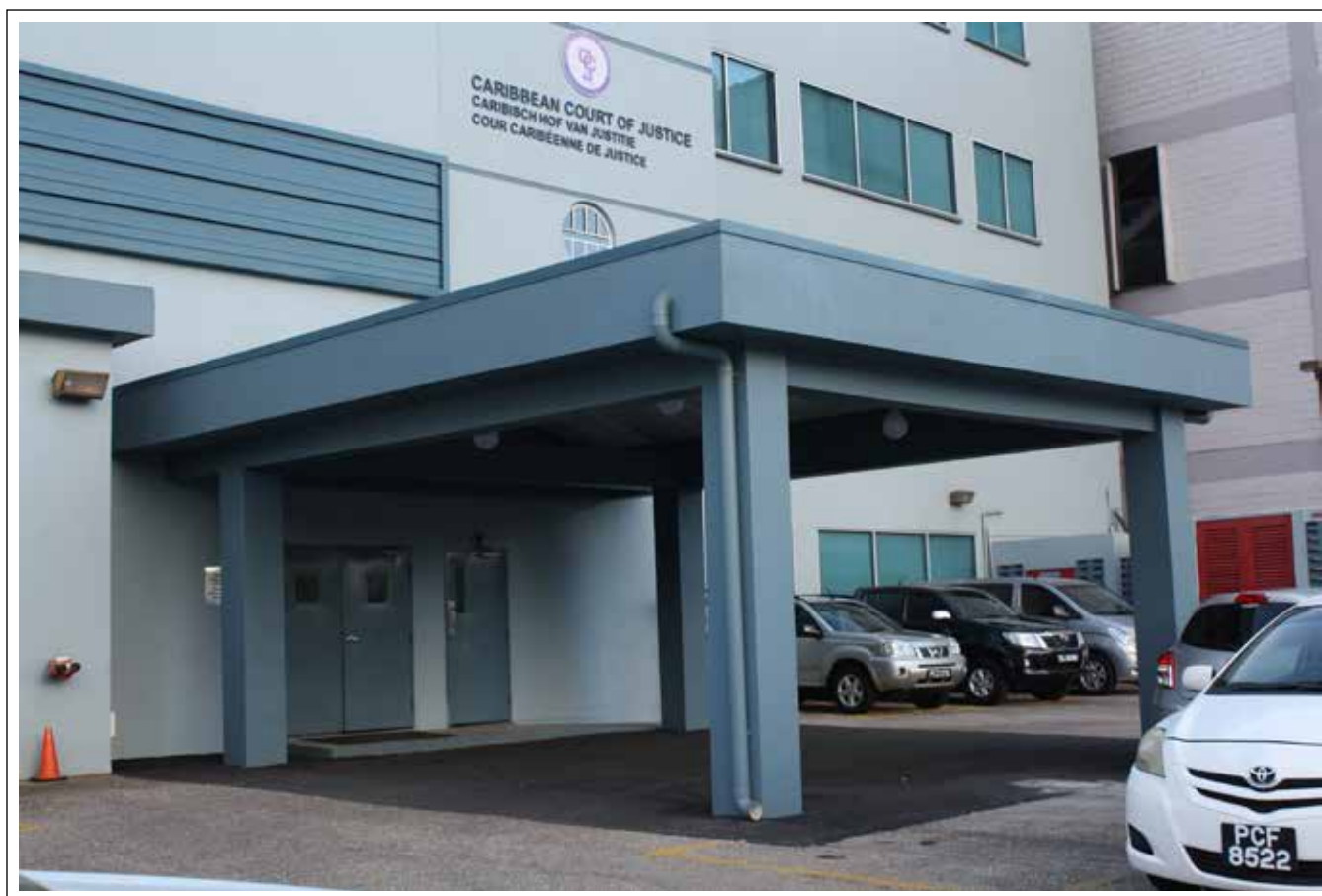
During the period under review, the Facilities & Assets Management Unit undertook a major project to supervise the construction of a new canopy at the rear of the Court’s building and a facelift to modernize the look of the building. The renovation was undertaken by the owner of the building, Hadeed and Hadeed, in collaboration with the Court.
